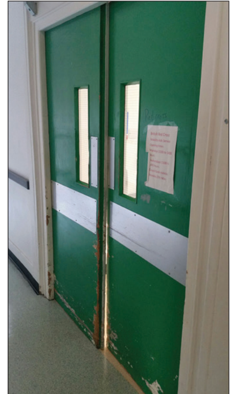
A familiar sight of an old doorset beyond its intended life with no potential for remediation.
