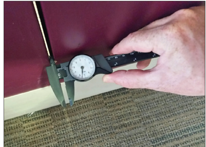
Checking a double door meeting gap with dial calipers during a Type 2 inspection.
