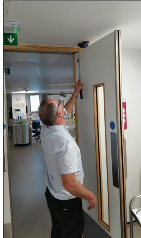
Checking the top edge of a door leaf during a Type 1 inspection Image courtesy of Golden Thread Fire Delay
