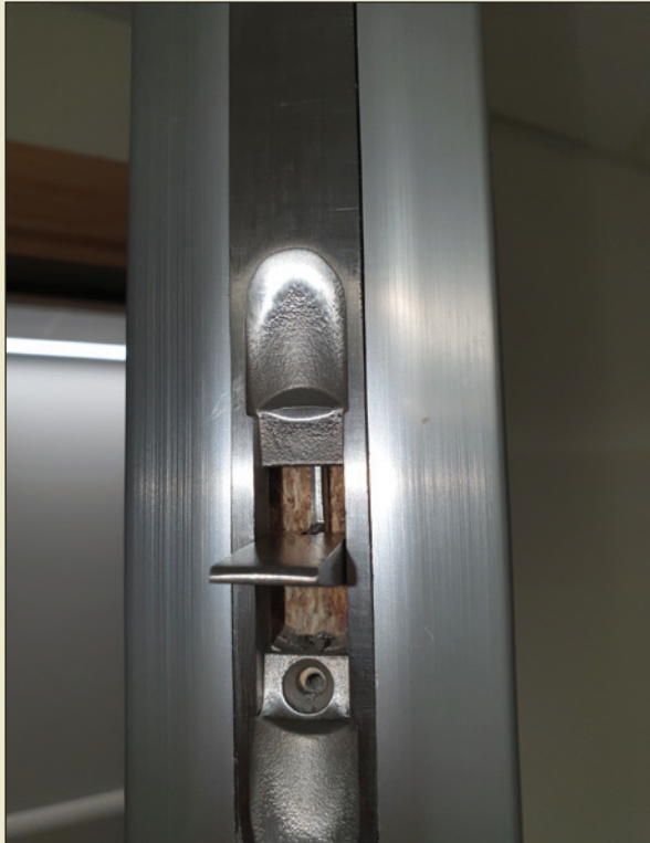
An example of missing intumescent protection to essential ironmongery.
