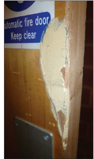
An extreme example of a door leaf in need or replacement.
