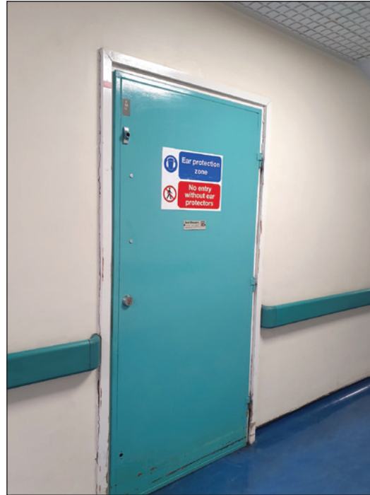
Image courtesy of Assured Fire Door Services
